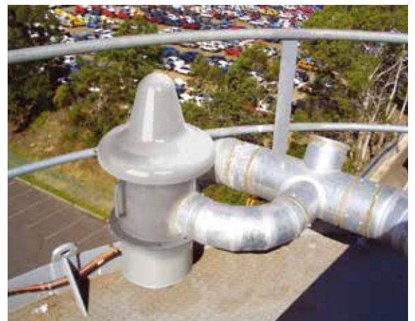
Silo workspace using VHS valve
